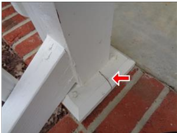
2.0 Picture 7 The split base plate for the left rail for the front steps.
