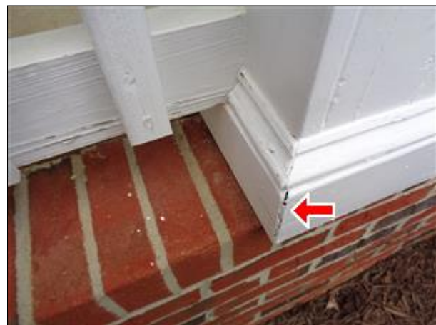
2.0 Picture 6 One of the cracks at the base trim for the column.
