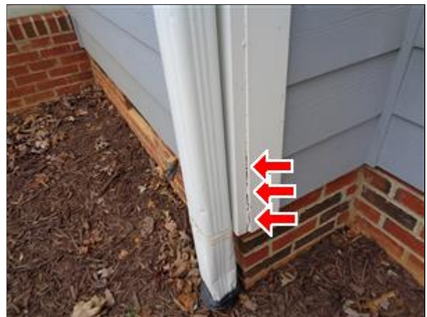
2.0 Picture 4 The crack at the corner board.
