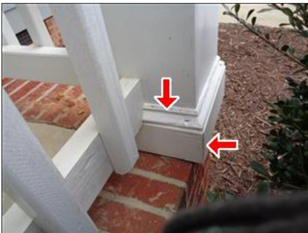
2.0 Picture 5 The deteriorated trim and crack at the joint at the right front column.
