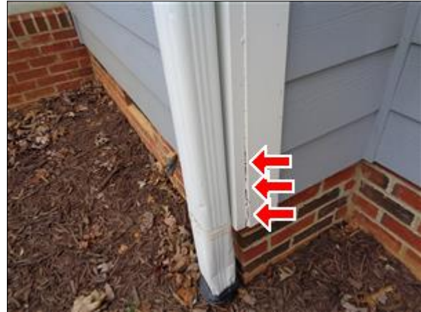
2.0 Picture 4 The crack at the corner board.
