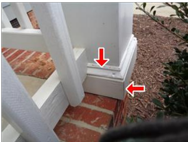
2.0 Picture 5 The deteriorated trim and crack at the joint at the right front column.
