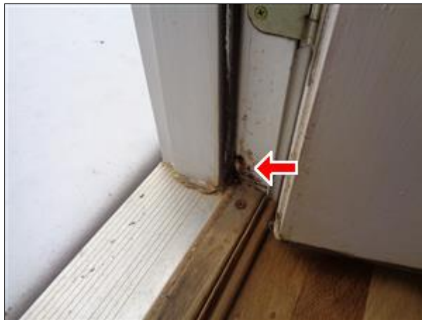
2.1 Picture 1 The deteriorated in the back door jamb.
