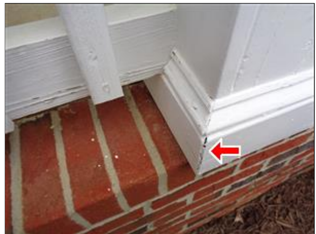
2.0 Picture 6 One of the cracks at the base trim for the column.
