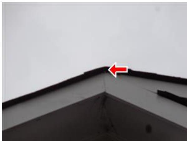
1.0 Picture 1 The broken place in the shingle.
