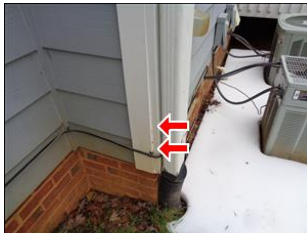
2.0 Picture 8 The cracked caulking.
