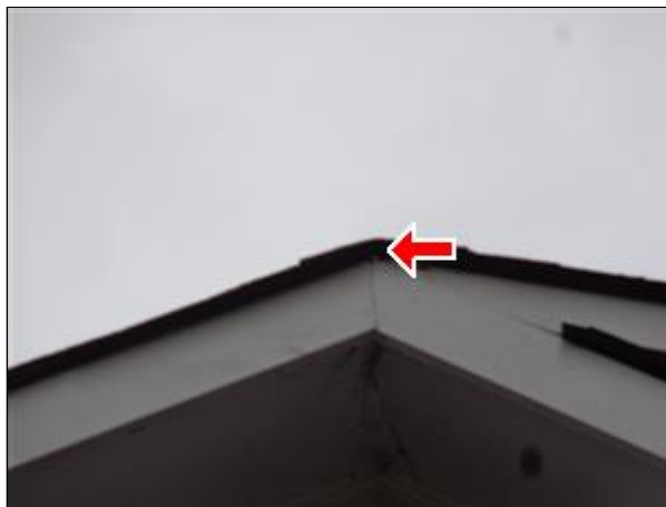
1.0 Picture 1 The broken place in the shingle.
