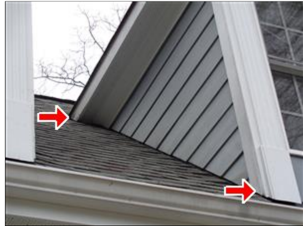
2.0 Picture 2 The left side of the left dormer.
