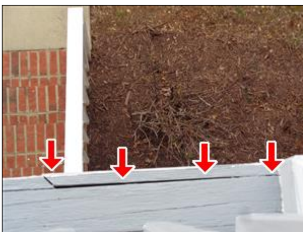
2.0 Picture 9 This is one area of the board across the front of the porch.
