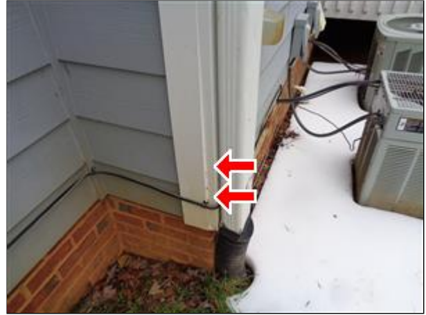
2.0 Picture 8 The cracked caulking.
