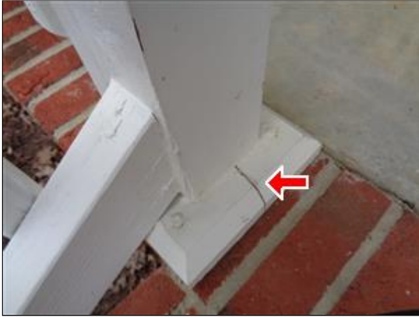
2.0 Picture 7 The split base plate for the left rail for the front steps.
