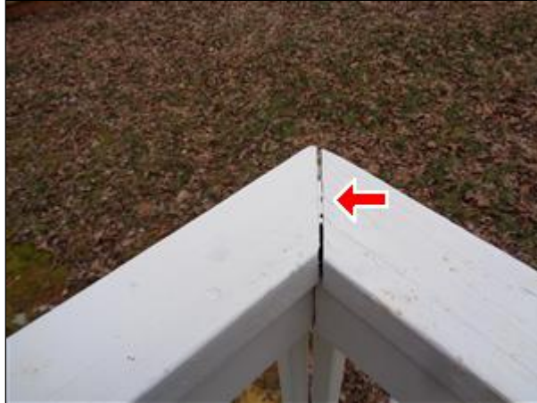
2.3 Picture 1 The crack at the corner of the top rail for the deck.
