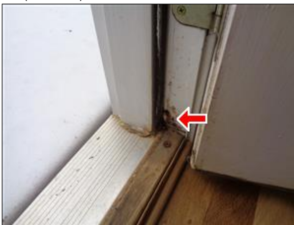
2.1 Picture 1 The deteriorated in the back door jamb.
